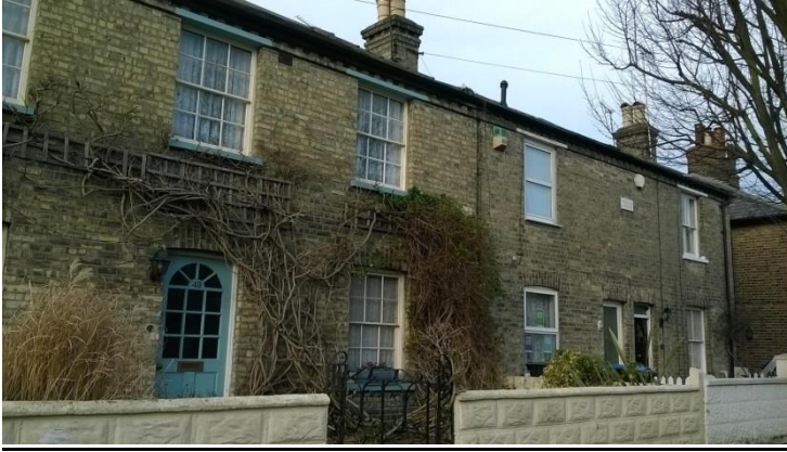
Figure 2: Timber six-pane sashes next to inappropriate uPVC windows
